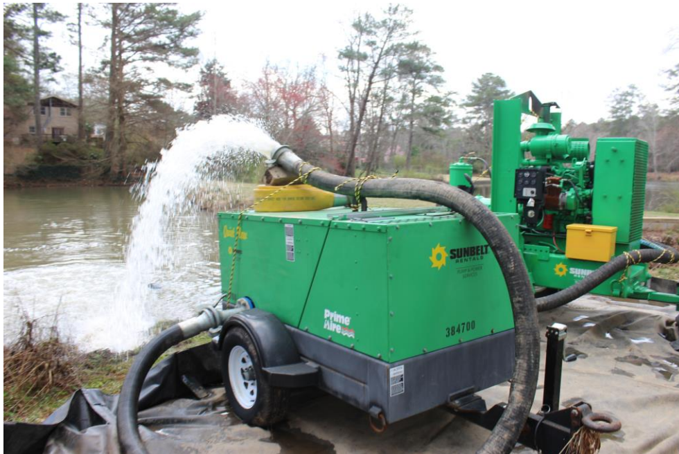
A pump aerates a Clarkston lake to restoring oxygen after a recent sewer spill.
