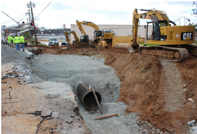
Crews completed work on a broken water main a day ahead of schedule.
