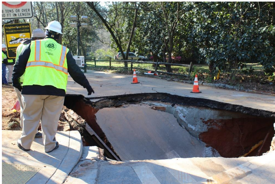
Crews are assessing the damage at a water main break.
