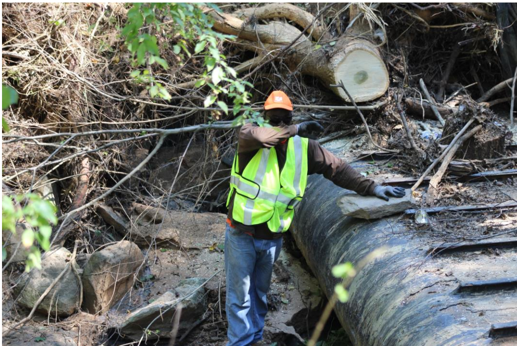
The large tree shown above was growing out of a concrete sewer box, causing the Aug. 23 spill into Snapfinger Creek.
