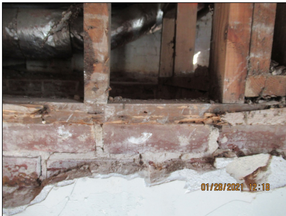
Photo 09: Decayed plate and studs. Typical throughout the basement.
