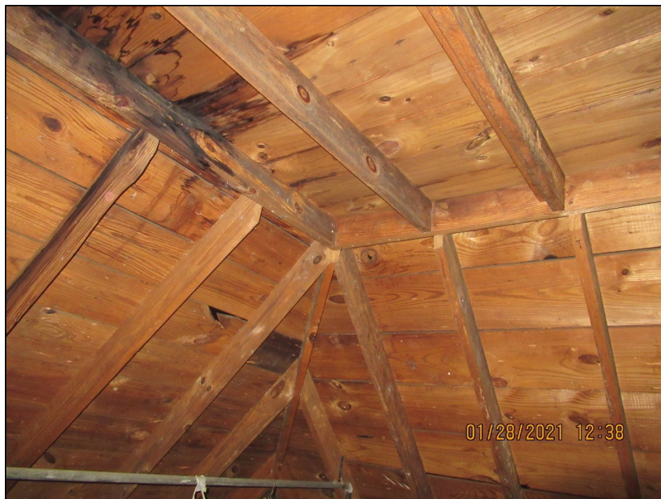
Photo 27: The flat roof is missing posts, adequate perimeter beam, connections for the flat rafters and the sloped rafter end cuts are greater than the ridge.
