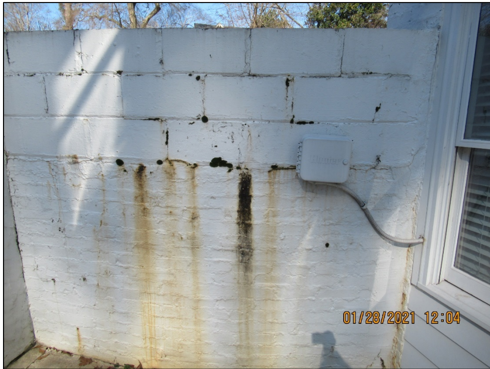
Photo 31: Failing retaining wall at the right side of the house.
