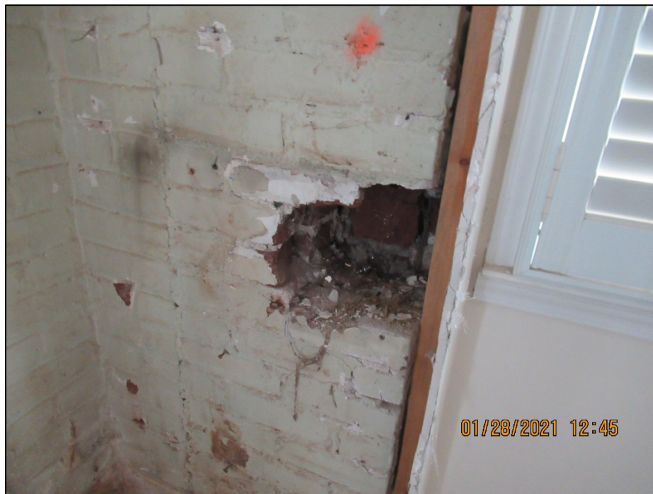
Photo 19: Damaged foundation wall.
