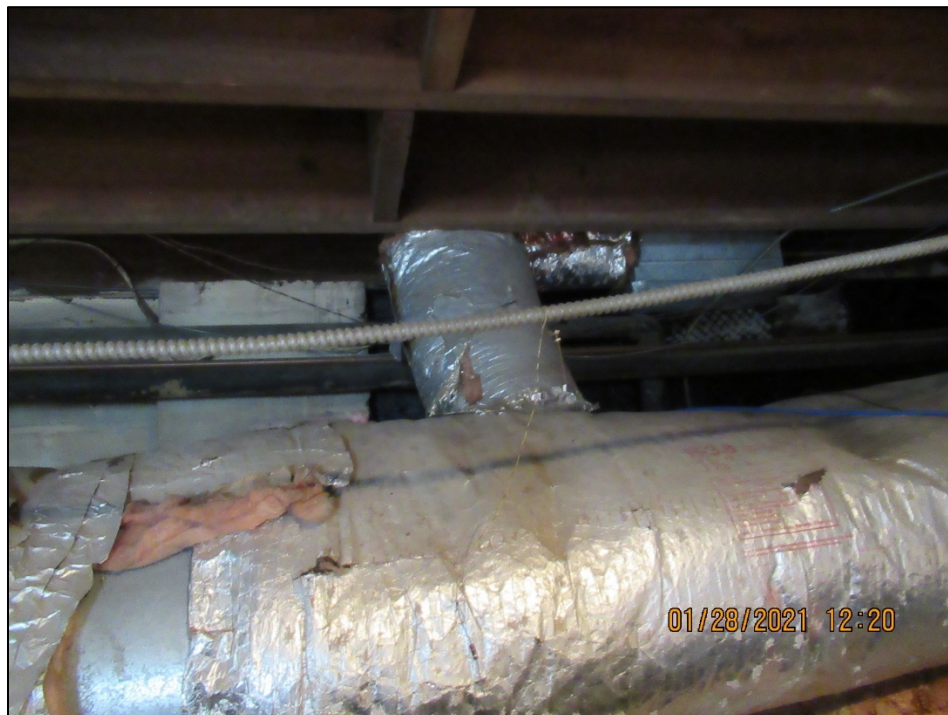
Photo 12: Poorly maintained HVAC ductwork, and the ducts are resting on the exposed earth.
