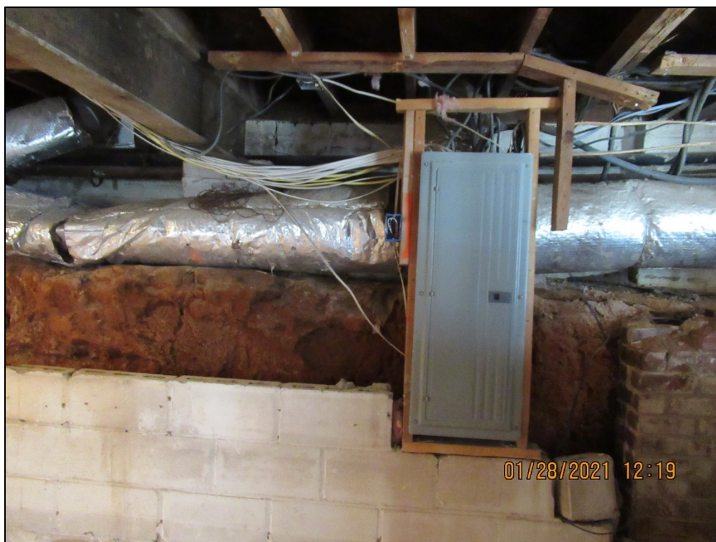
Photo 10: The electrical panel was next to the earth cut, supported by a failing retaining wall and decayed studs.
