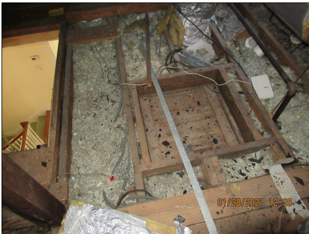
Photo 29: Inadequate ceiling insulation.
