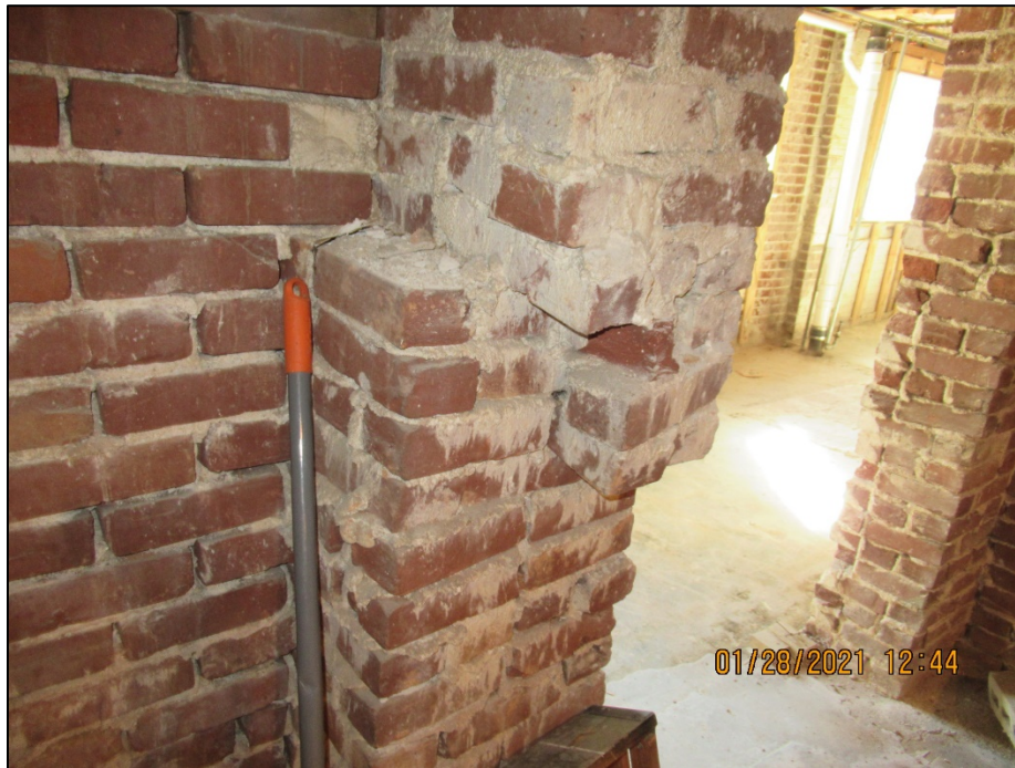
Photo 18: Missing brick for part of the foundation system.
