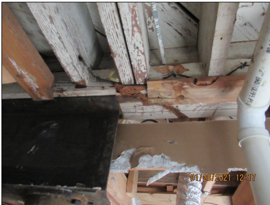
Photo 04: Typical decay and deterioration of a main beam for the first floor.
