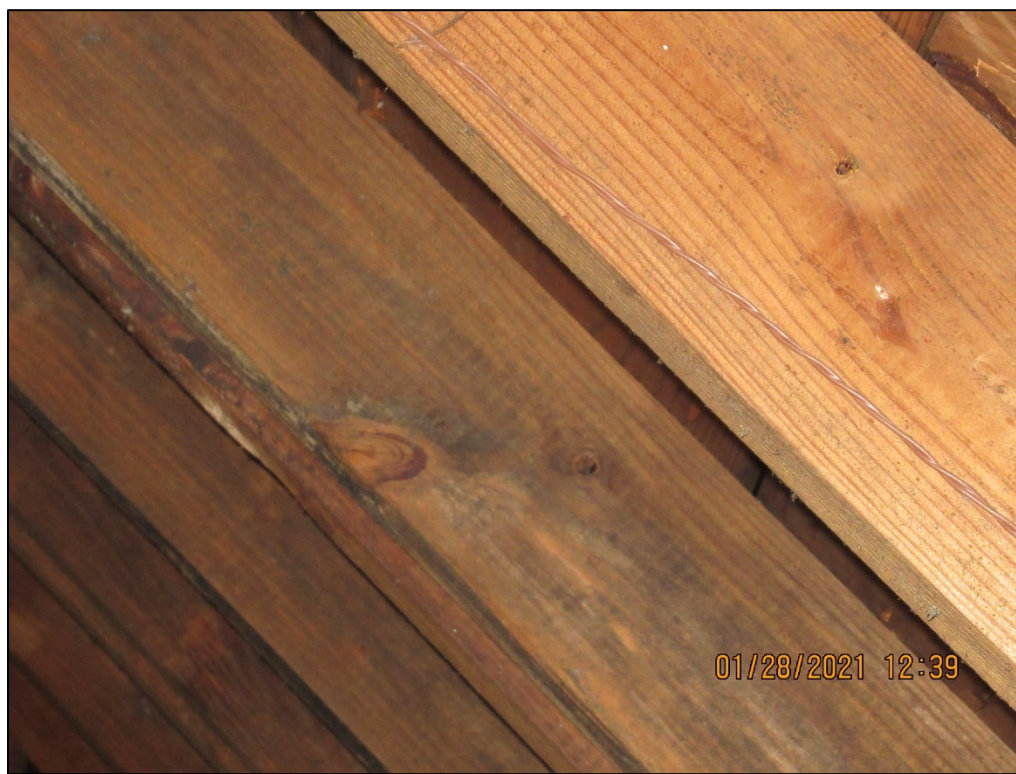
Photo 30: Typical splits in rafters caused by age and heat in the attic.
