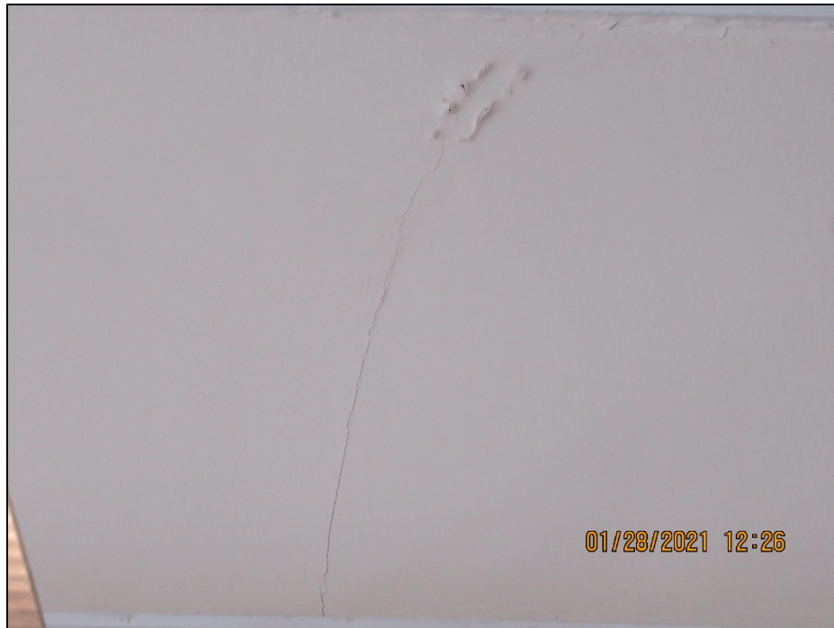
Photo 21: Typical Cracking and water damage at all of the first floor windows and door openings.
