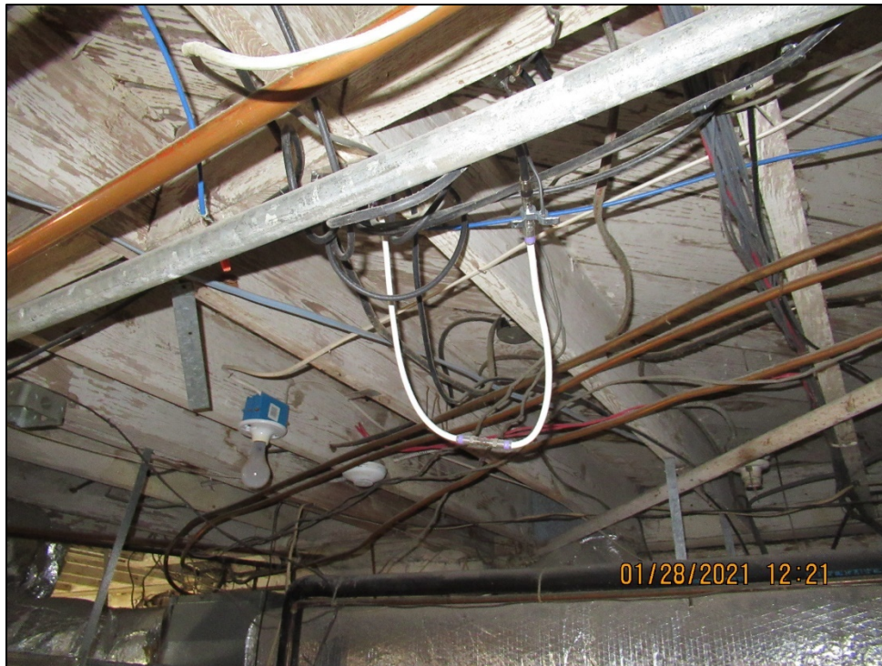
Photo 13: A jumble of electrical wiring.
