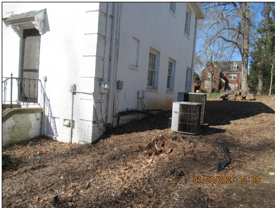
Photo 36: At the left side, the grade slopes toward the house and it appears to be above the foundation wall.
