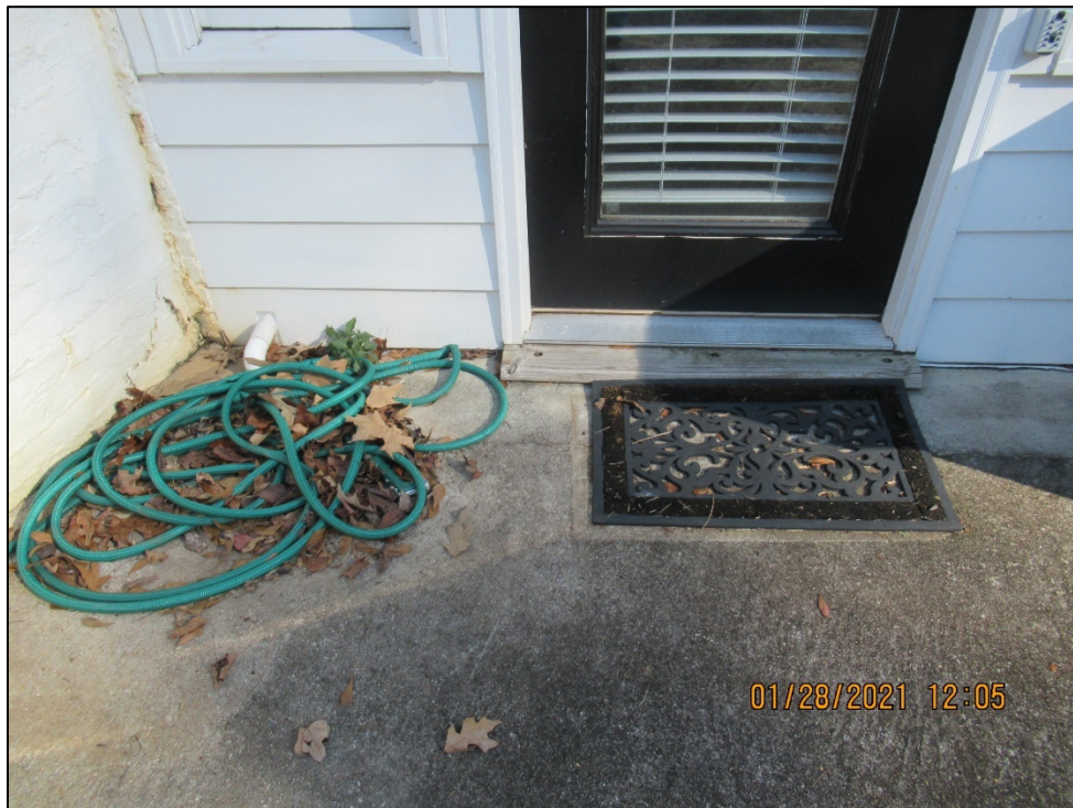
Photo 32: The driveway was placed too high exposing the basement to water infiltration. Note the modern siding and doors.
