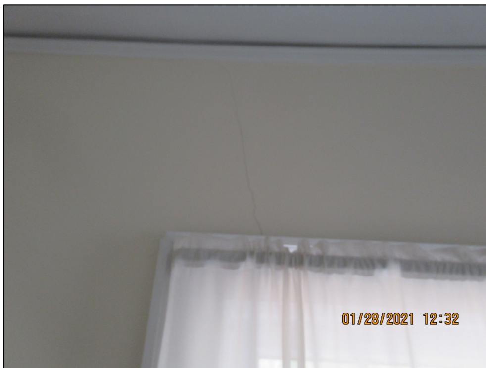
Photo 26: Typical cracks at the windows and doors for the second floor indicating movement of the structure.
