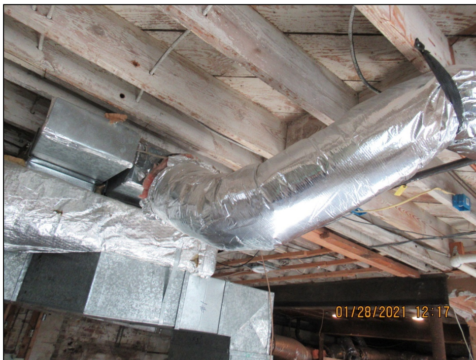
Photo 03: HVAC ductwork that was not insulated and in poor condition. Some of the ductwork had been replaced.
