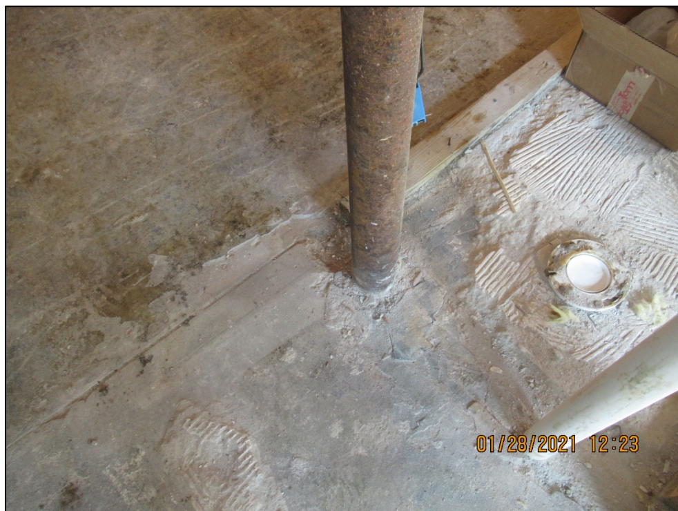
Photo 17: Corroded support posts.
