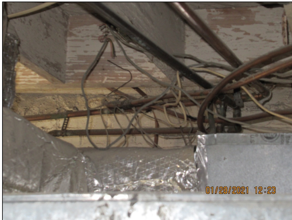
Photo 14: Another jumble of electrical wiring touching the copper plumbing pipes.
