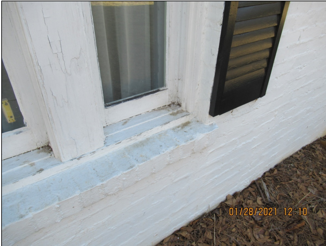
Photo 37: Typical window that has decay at the frames and sill.
