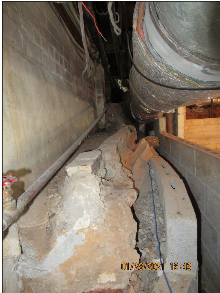
Photo 20: Failing 4" CMU retaining wall near the front foundation wall.
