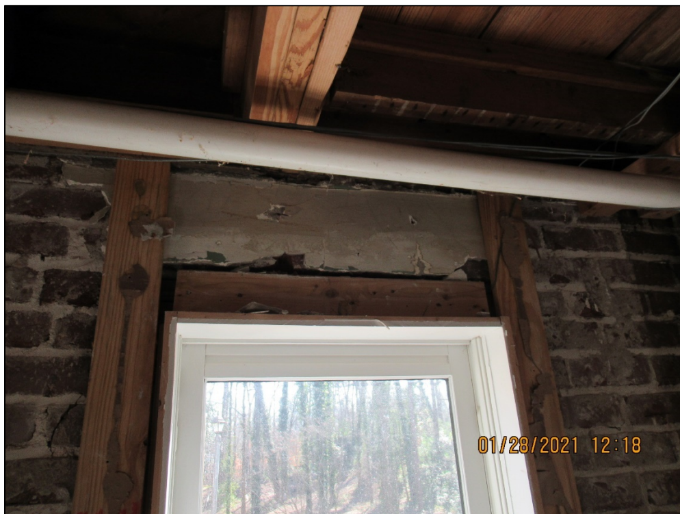
Photo 06: Damaged concrete and wood header at basement window
