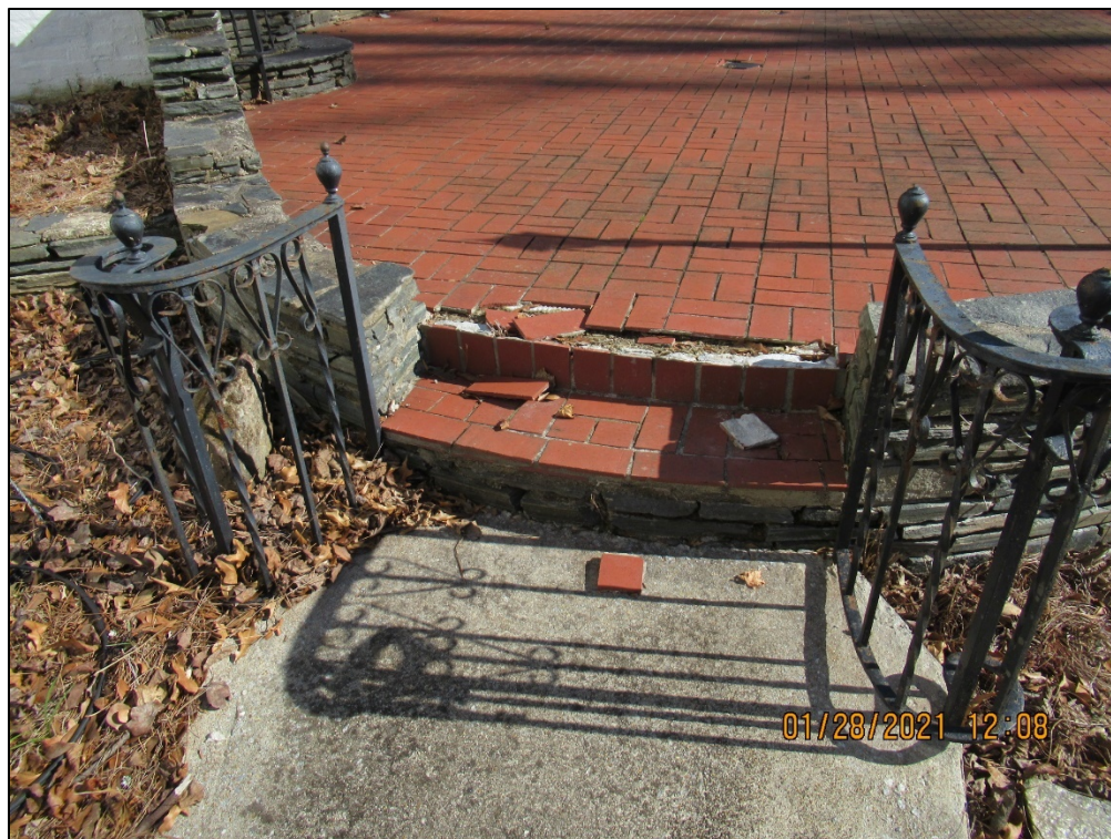
Photo 33: The patio had many issues such as settlement and paver deterioration.
