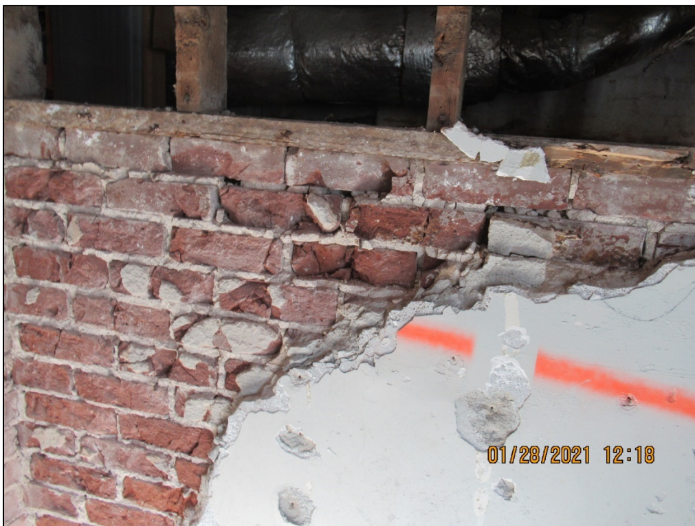
Photo 08: Deterioration of foundation wall that is part of the crawl space. Note the decayed wood plate on top of the wall.
