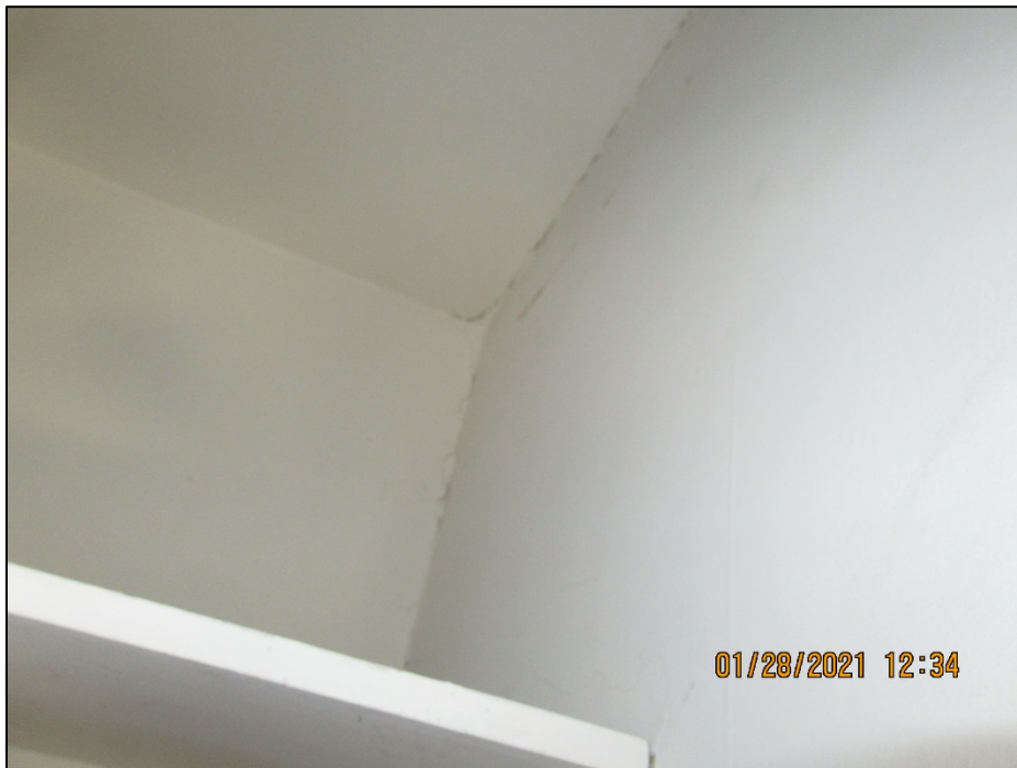
Photo 22: Cracks and water damage in first floor closet.
