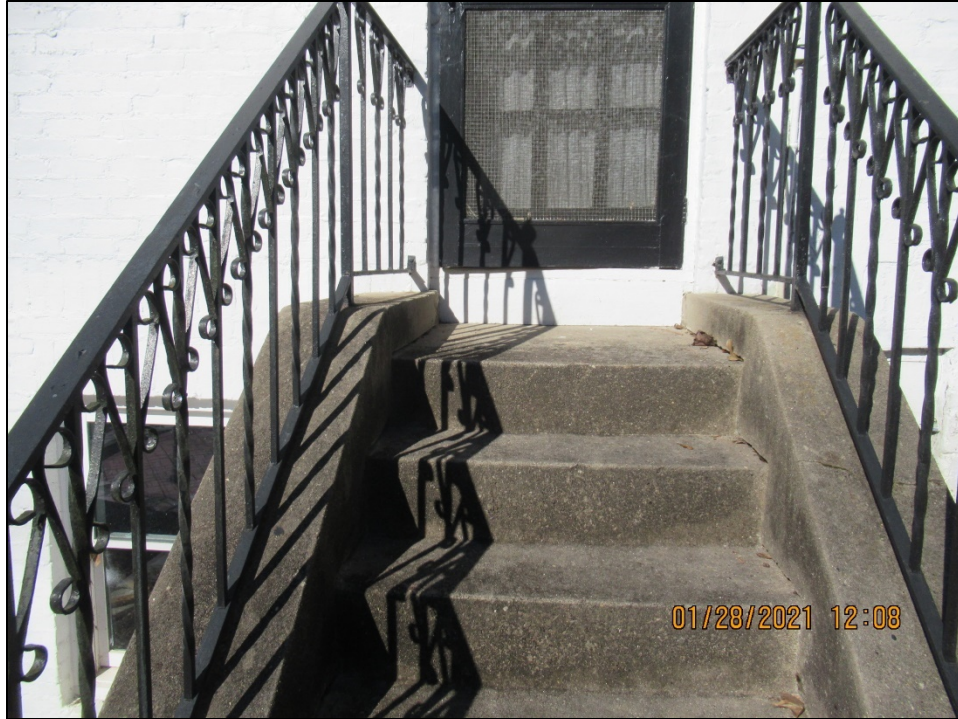
Photo 35: The stairs at the rear of the house do not have an adequate landing at the top and bottom of the stair flight. The risers are too high.
