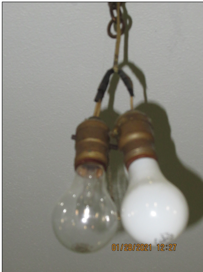
Photo 24: Original wiring for the house.
