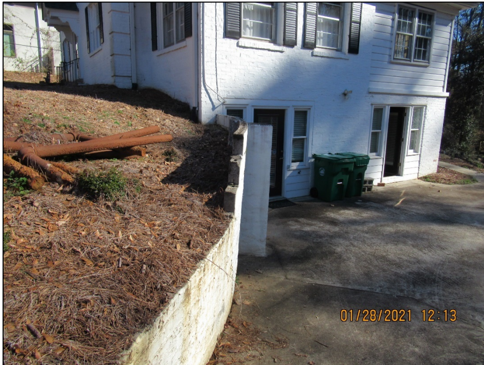
Photo 02: View of the right side of the house. Note the leaning retaining wall.
