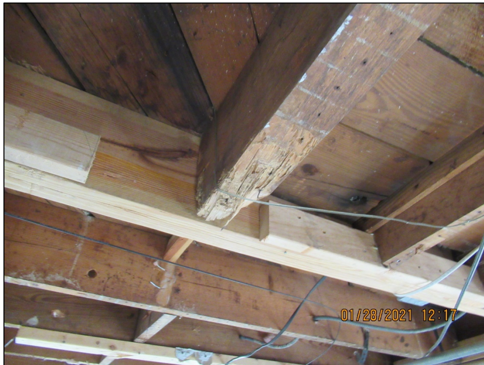
Photo 05: Damage to a main beam for the first floor.
