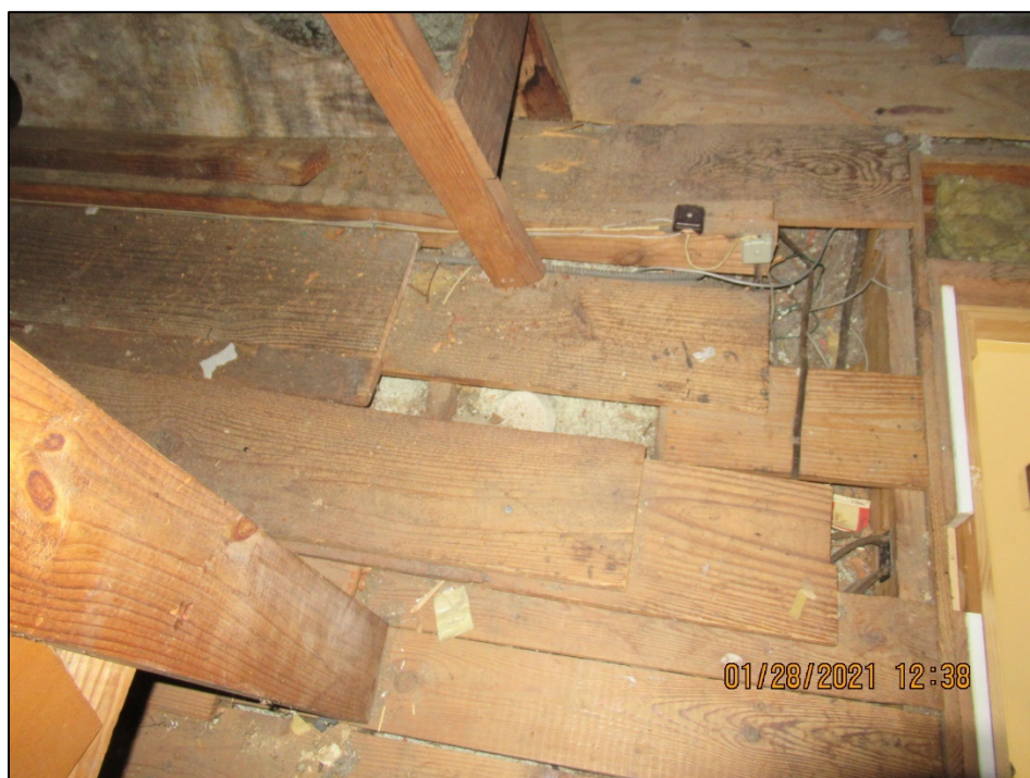
Photo 28: Missing decking that is a fall hazard.
