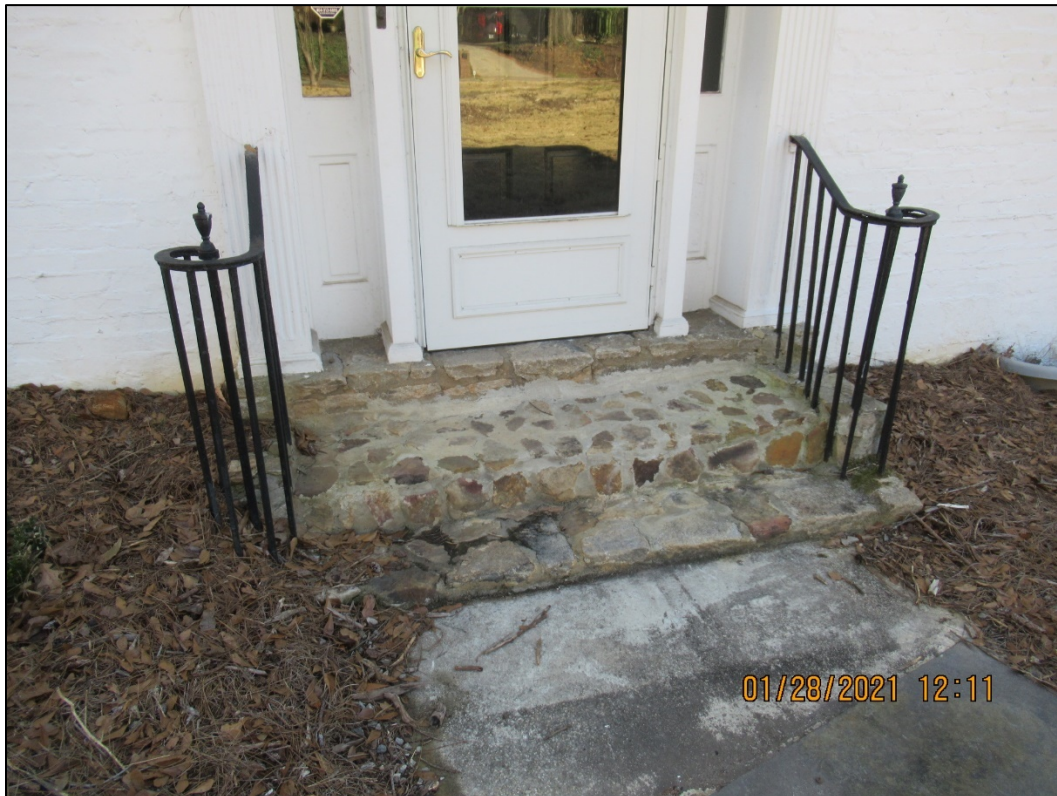
Photo 38: The landing at the front door does not comply with the code requirements for depth. The bottom step has deteriorated.
