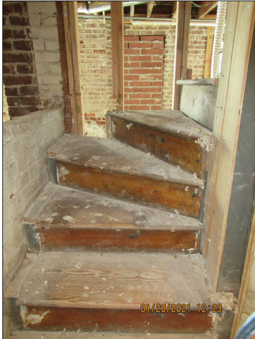
Photo 15: The stairs from the basement to the first floor. All of the stair components do not meet the IRC requirements.
