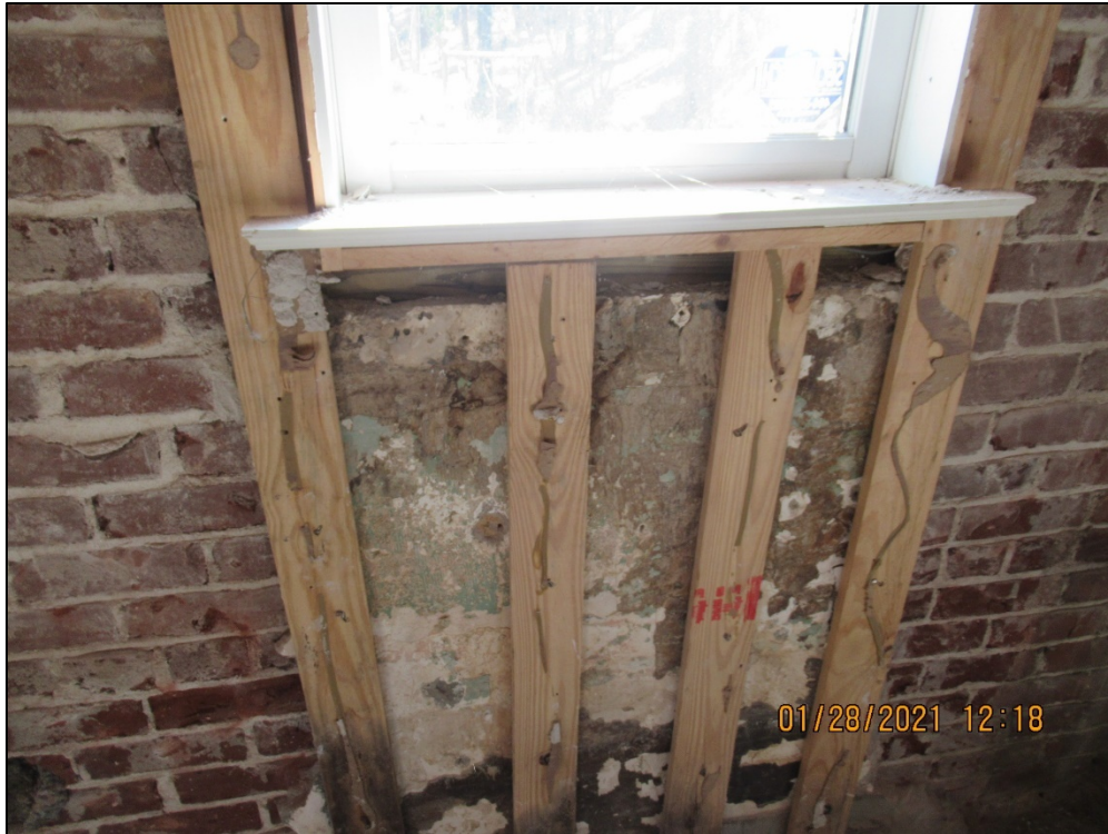
Photo 07: Decayed wood at window.
