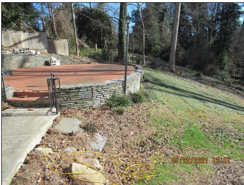
Photo 34: The patio retaining wall is failing.
