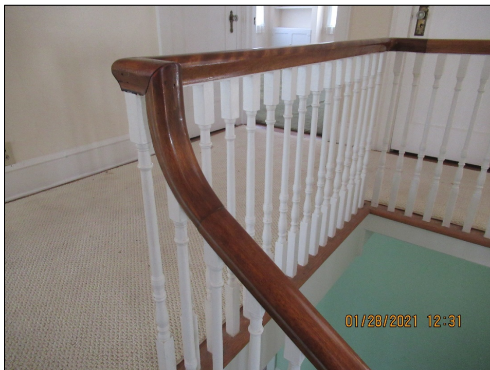
Photo 25: The guardrails do not have the minimum 36" height as required by the code and they are a safety hazard.
