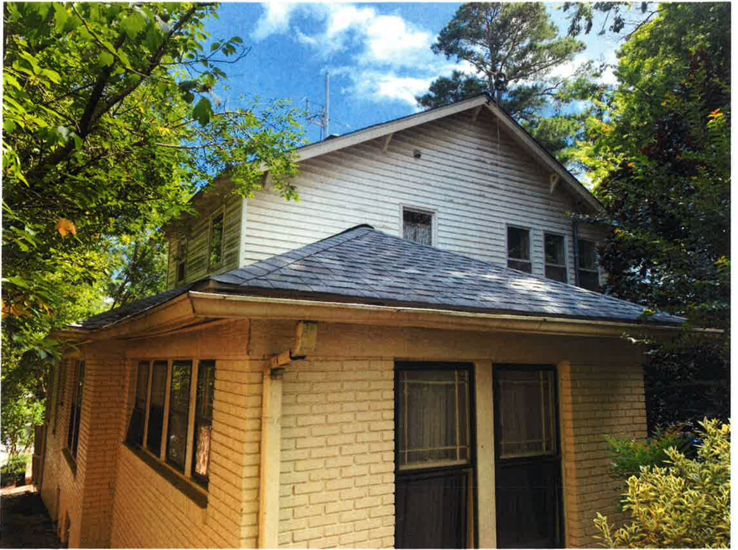
Figure 2: View of vinyl siding and windows on second floor addition as seen from back yard (Not visible from street)
