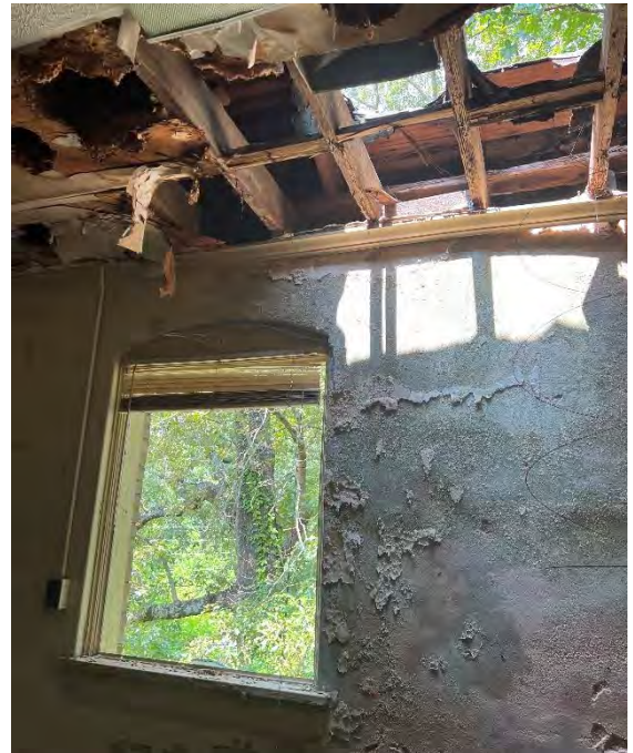
IMG CH3-2: Hole, one of two, in roof allowing structural deterioration. Framing repairs needed before roof replacement.
