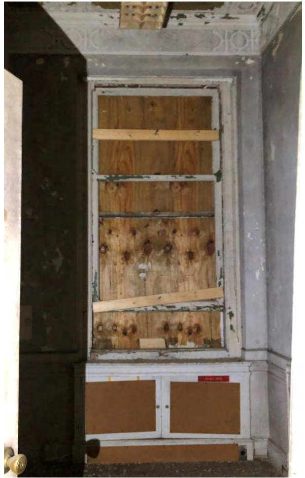
IMG 111-2: The space is currently divided up into various office spaces used in the institution era. This wood window will be removed to create an opening to a new LULA elevator in Lightwell 1.
