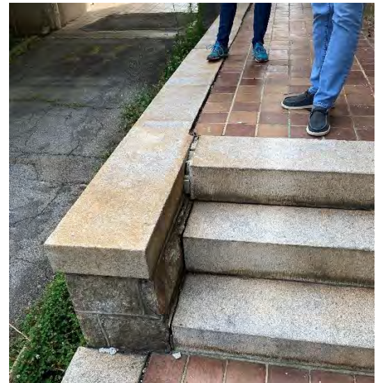
IMG EX6-6: Stone retaining wall breaking away from tile walkway; needs to be redone.
