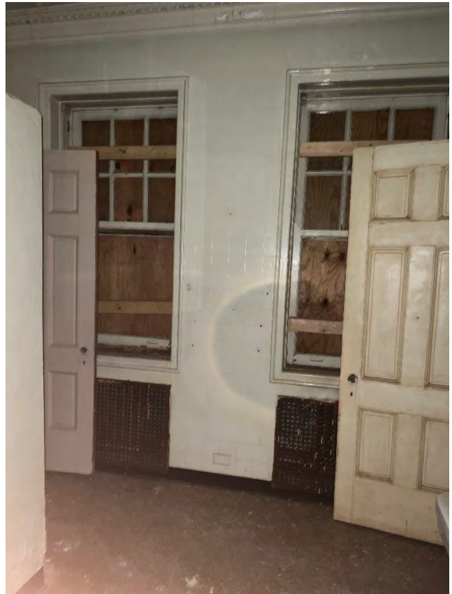
IMG 204-2: Recessed radiator enclosures with cast iron grilles below windows. Ornamental tile casing at windows and doors. Ornamental tile crown mouldings. (all with epoxy coatings to be removed)
