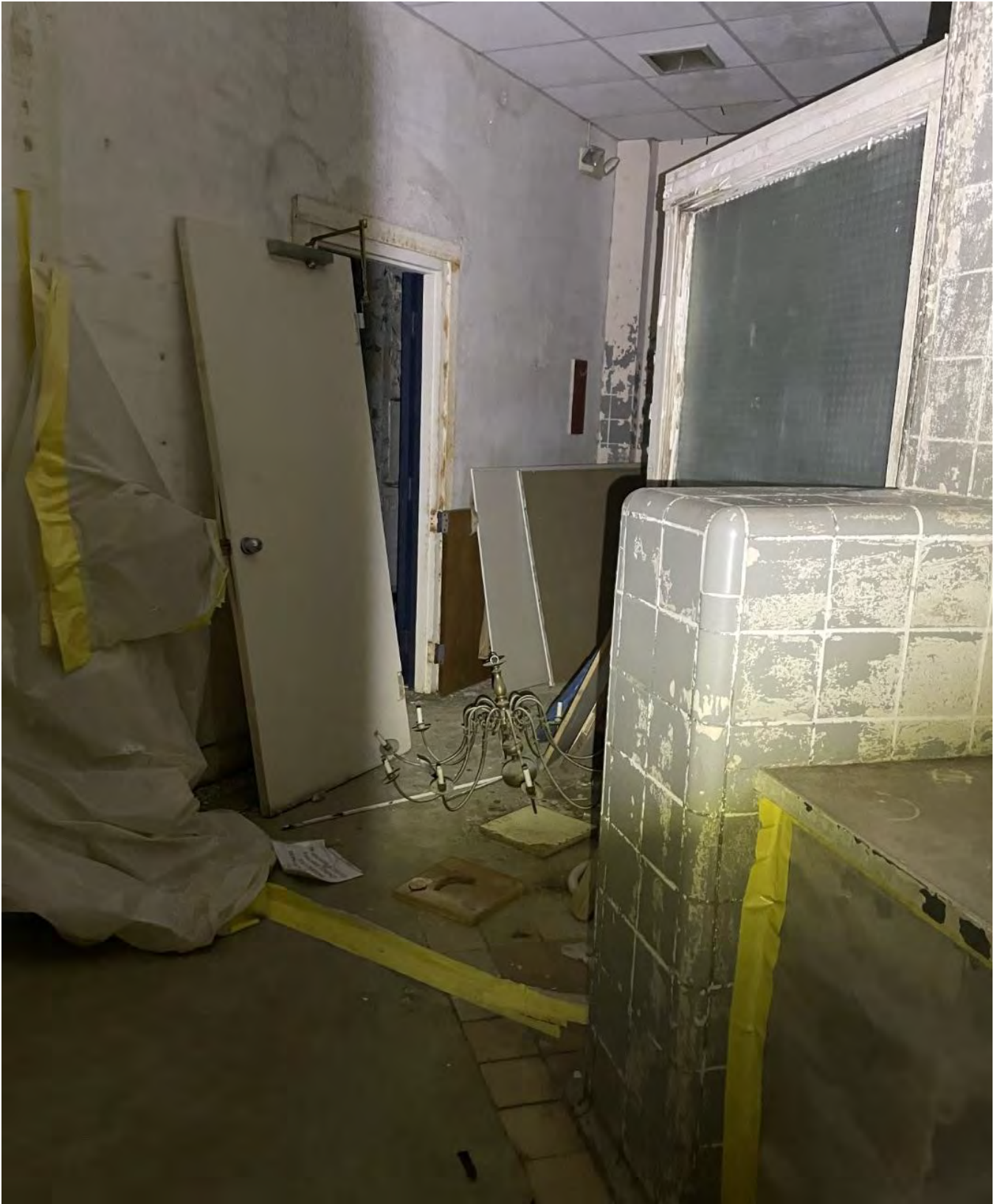
IMG 114-1: Original Kitchen was divided up into many rooms during the institution era. Tile @ floors, full height walls and even ceilings appear to be original materials. Area of mansion to contain new restrooms serving future event/assembly uses.
