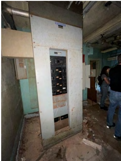
Figure 3: Existing Building Main Switchboard
