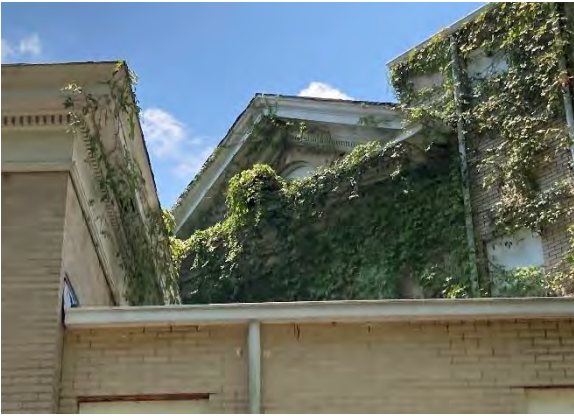
IMG EX6-1: Extensive overgrowth around the exterior. Here seen in Lightwell Two.
