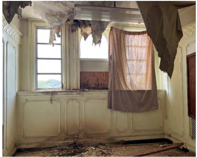
IMG 311-2: Water damaged plaster ceiling in South Alcove. Aluminum replacement windows to be removed and replaced with historically accurate wood sashes.
