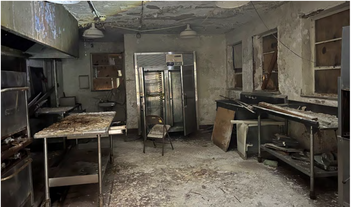
IMG 123-1: Institutional Kitchen addition off of the Banquet Hall in poor condition.
