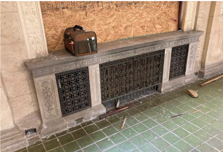
IMG 101-3: Cast stone radiator enclosures with cast iron grilles.
