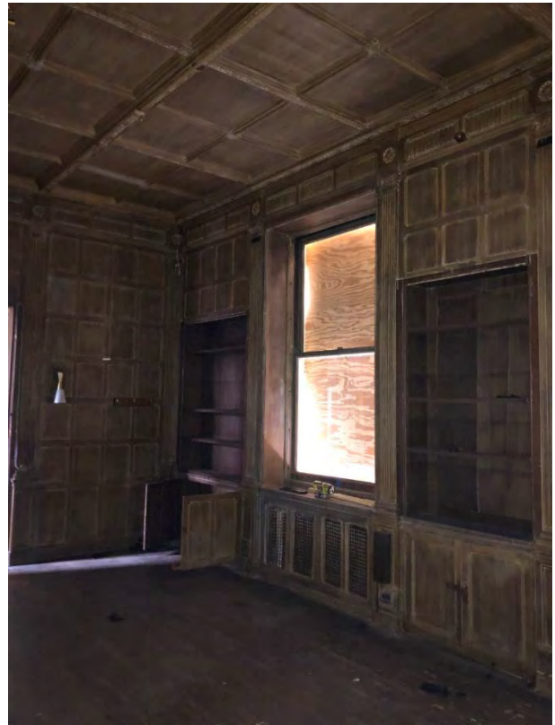
IMG 104-4: Built in shelves. Shelves at right in photo water damaged. Back of shelf to be replaced in-kind.
