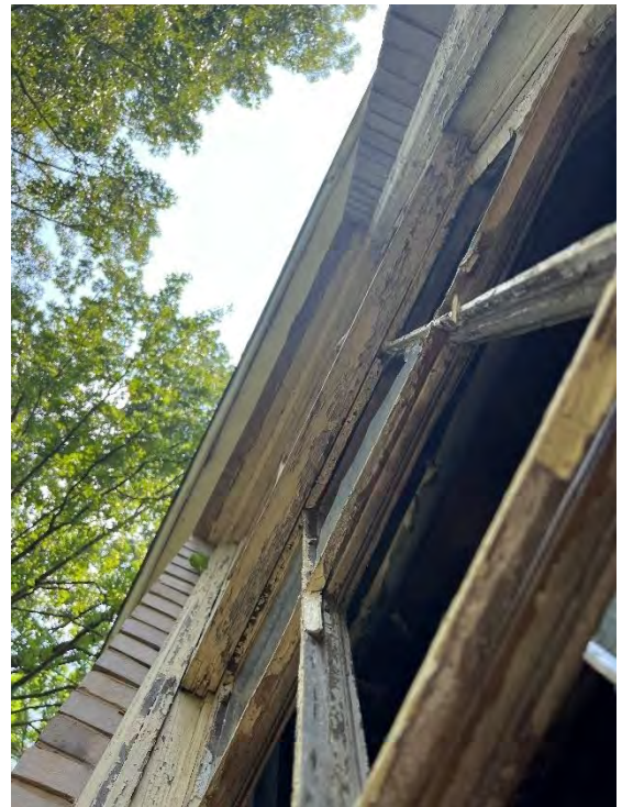
IMG CH3-5: Chipped paint and wood on windows. Window is missing windowpanes.
