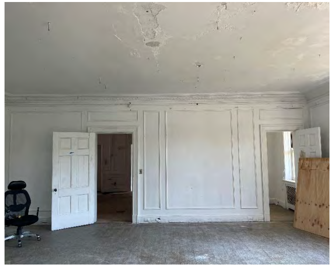
IMG 208-4: Typical smooth plaster walls with applied wood moulding creating panels. Looking north at doors leading to Stair Hall and Bath 4 & Closet. Typical ceiling damage visible after removal of ACT ceiling systems.
