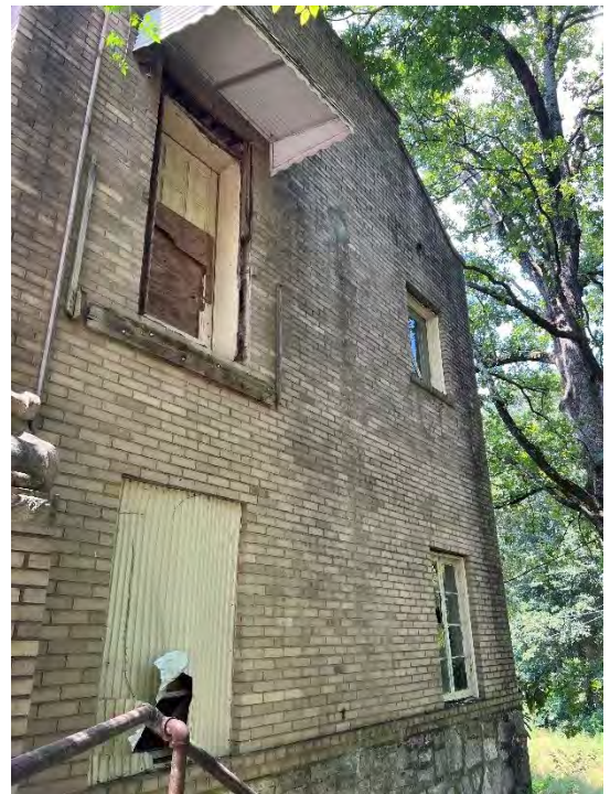
IMG CH1-2: North side with stairway down to back of Carriage House. Replace door with window matching adjacent.
