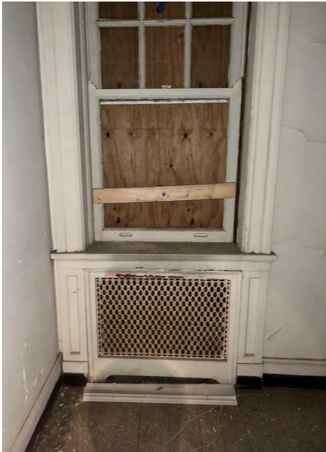
IMG 206-1: South Hallway with typical radiator enclosure as seen in most of the mansion. (this window was originally in end bedroom on this wing but became part of egress corridor when stair was added to end of wing.)
