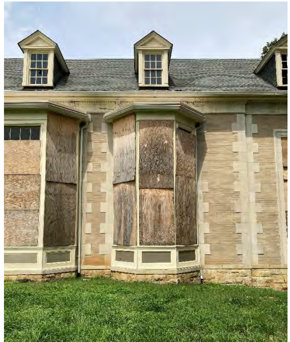
IMG EX4-2: Boarded up, damaged windows of the Music Room.
