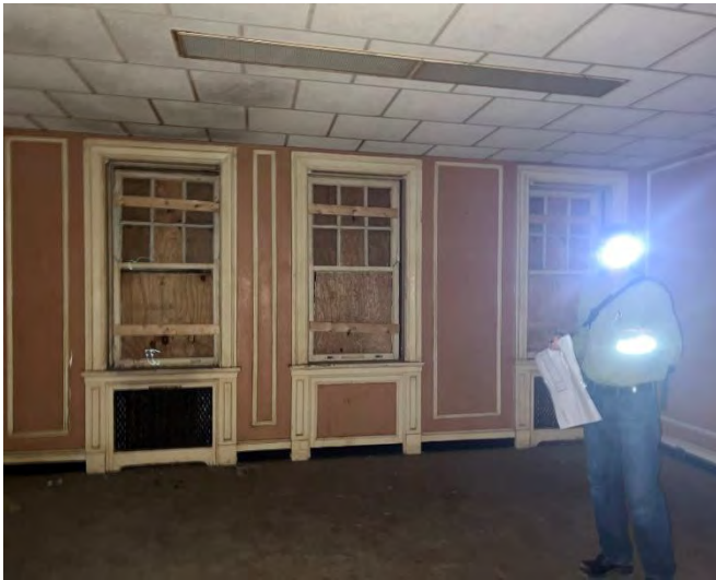
IMG 203-1: Typical bedroom on the second floor of the mansion. The radiator enclosures are typical for most of the enclosures throughout.
