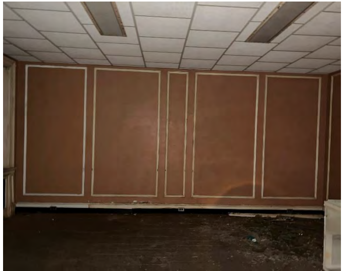
IMG 203-2: Paneling on the walls and crown molding hidden by institutional installation of ACT ceilings in all second-floor rooms and wing corridors.
