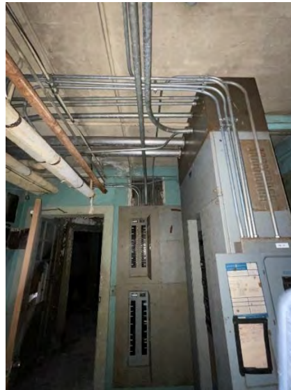
Figure 4: Branch circuit panelboards on Basement Level
