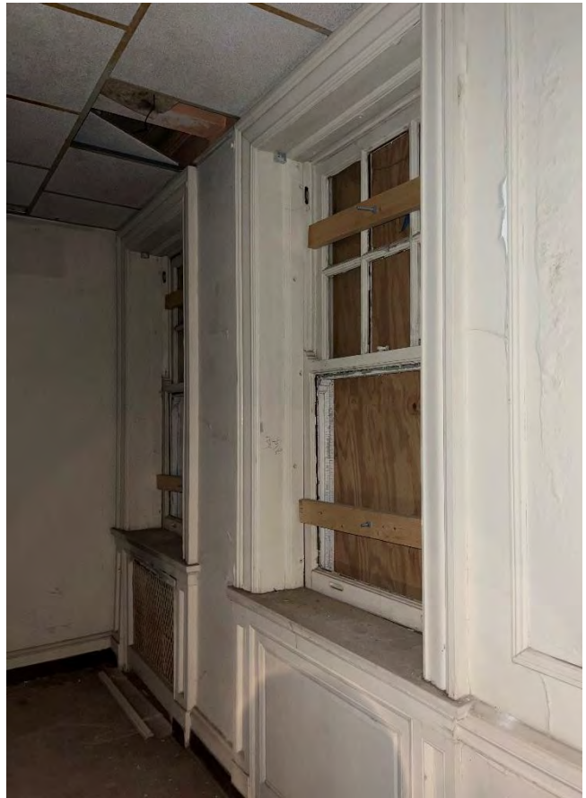
IMG 206-2: South Hallway paneled wainscot and wall panel molding. Glazing “removed” at majority of windows to install exterior plywood security coverings.
