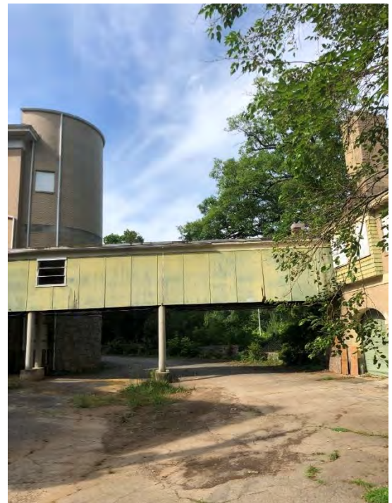
IMG CH1-5: Bridge connection from Main House to Carriage House which is to be demolished.
