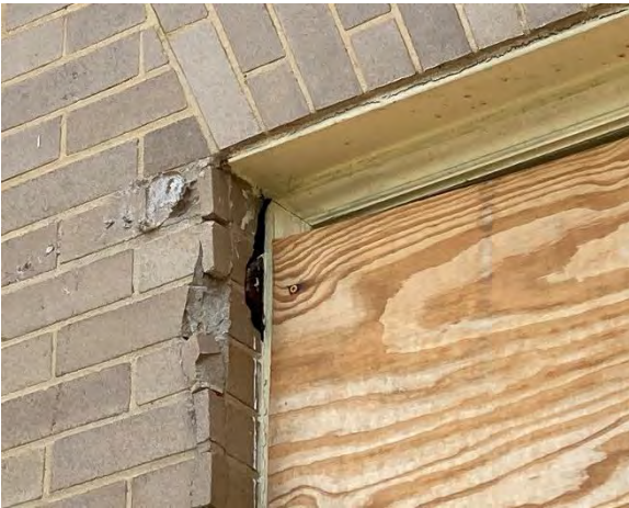
IMG EX6-3: Crumbling wood on the top corner of a jack arched window.
