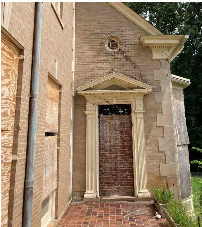
IMG EX4-3: Detailed trim of brick-filled door that leads to nothing on the interior side. Trim needs repair.
