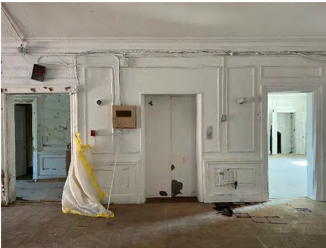
IMG 209-3: Elevator installed at former Bedroom closet location on this floor. Door on left leads into Back Stair Hall and North Hallway. Both with severe water damage to plaster and wood paneling finishes.
