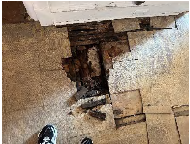
IMG 209-4: existing ACT flooring on plywood installed over original tongue and groove wood flooring. Areas of water damage revealing layers shown here.
