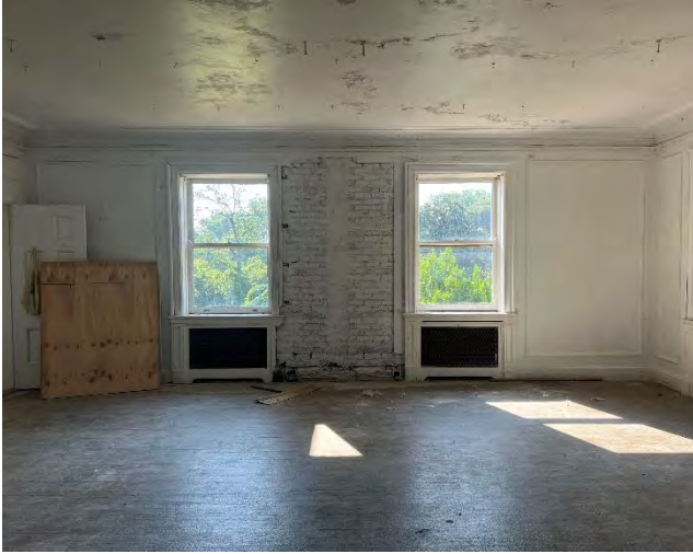
IMG 208-1: Candler's bedroom which showcases water damage on the front side of the mansion in between two windows.
