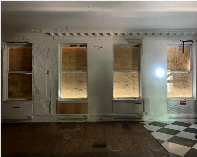
IMG 102-1: Family Living Room with water damage located on the left side of the image, effecting both the wall and ornate plaster crown molding with corbels. Tile floor section not original. 1 ½" T&G oak typical at Main House 1 st Floor
