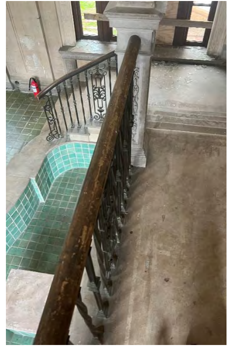
IMG 101-2: Concrete stairs and original railing leading down into Solarium. Fountain element integrated into stair design.
