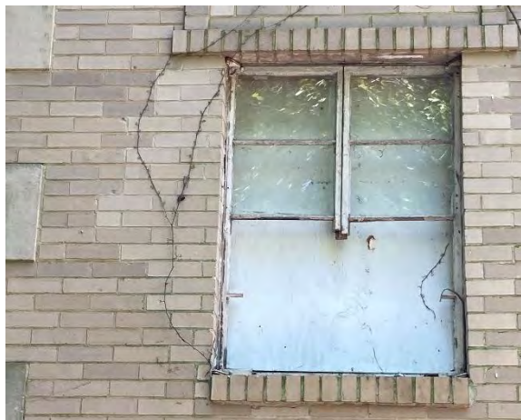
IMG EX6-5: Broken steel window on the Organ Room; typical for many steel and wood windows around the property.
