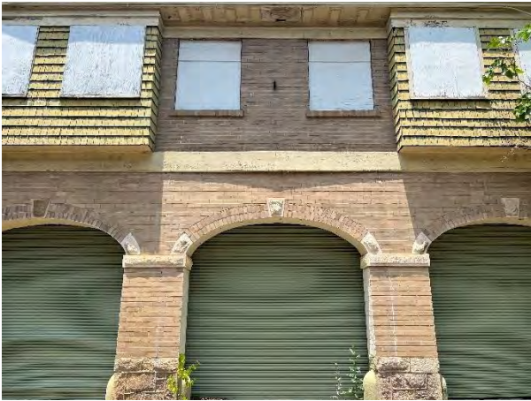
IMG CH1-1: East facing, front portion of Carriage House. Deteriorating roof trim and paneling need to be fixed.
