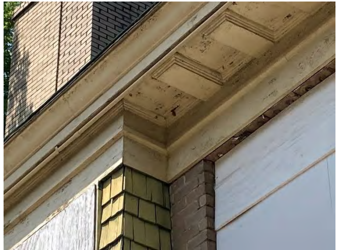
IMG CH2-4: Corner where deteriorating paneling connects with trim as well as brick wall.
