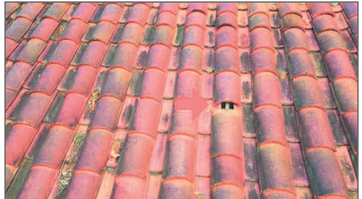
2. Damage, missing, loose, torn
