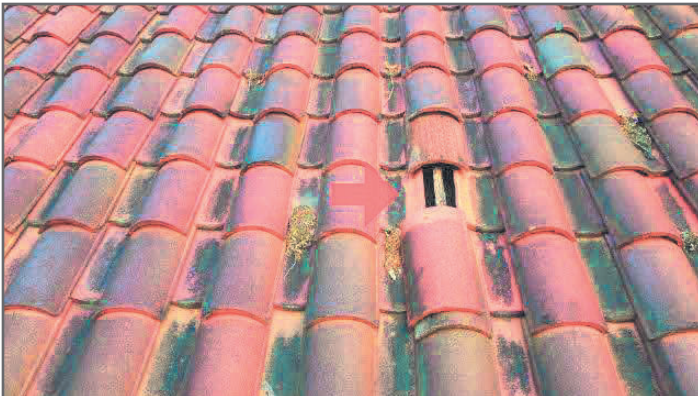
1. Damage, missing, loose, torn
