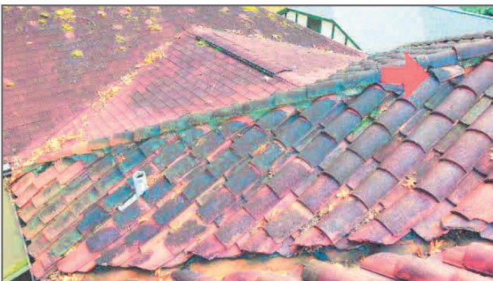
3. Damage, missing, loose, torn
