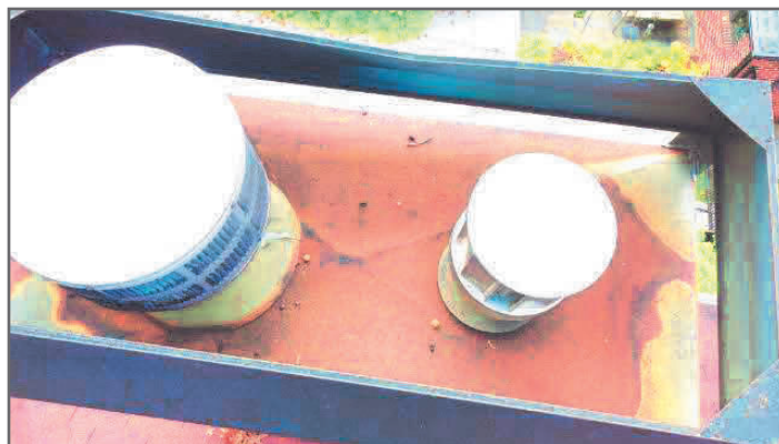
12. Chimney cap rusted or ponding
