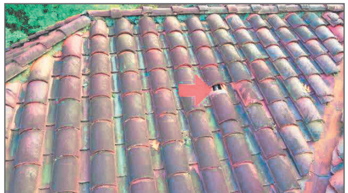
4. Damage, missing, loose, torn
