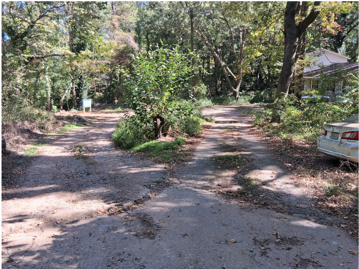
Kelly St. splits into two lanes, badly rutted, old gravel and asphalt.
