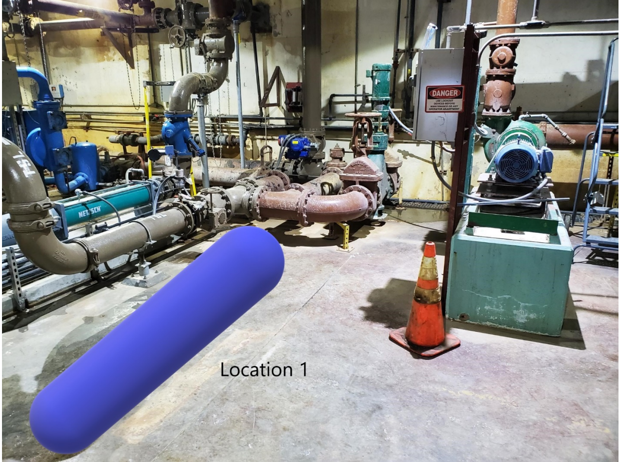
Current Netzsch pump in the background
