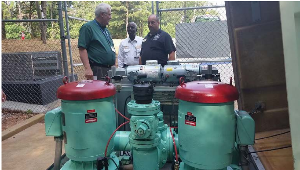
DeKalb officials inspect new upgrades that have the capacity to hold 750 gallons per minute of sewage
