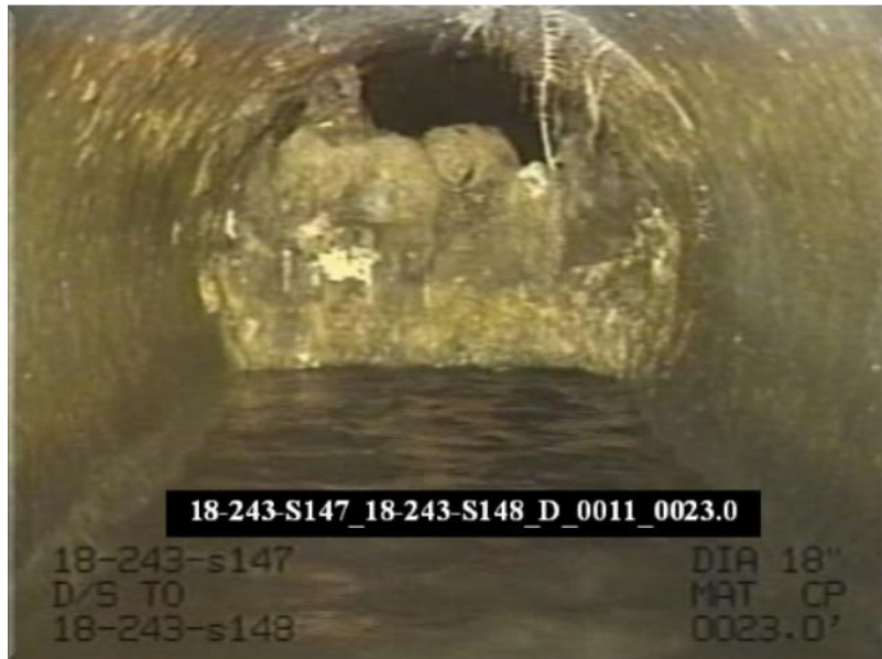
DeKalb County pipe clogged with fats, oils and grease.
