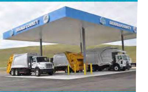
CNG Station - Seminole Road Landfill
