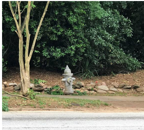
Fire hydrant located at Briarcliff Road and University Drive is the connecting point between two aging water mains that are contributing to low water pressure in the area.
